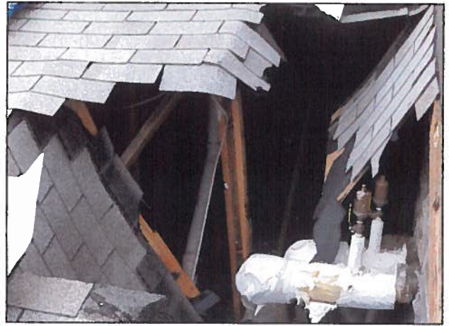
Photo 2: Masonry crashes through the roof following earthquake.
