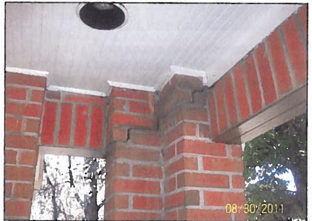
Photo 4: Masonry columns pulled away from an end wall.
