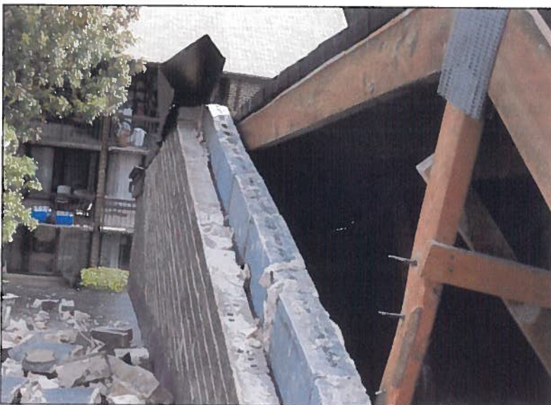
Photo 1: Masonry dislodged from a pitched roof truss.
