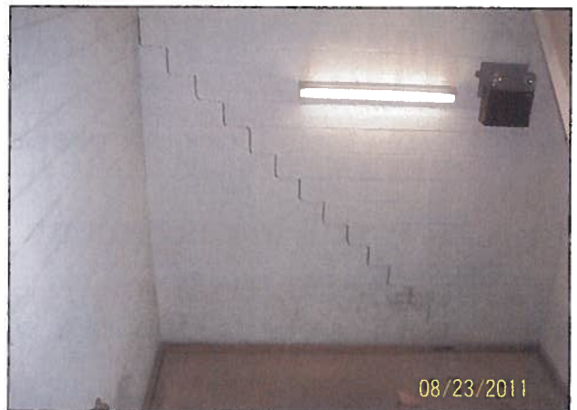
Photo 5: Rigid stairwell towers, used to stabilize the structure, cracked in sheer because they could not withstand the quake's lateral loads.
