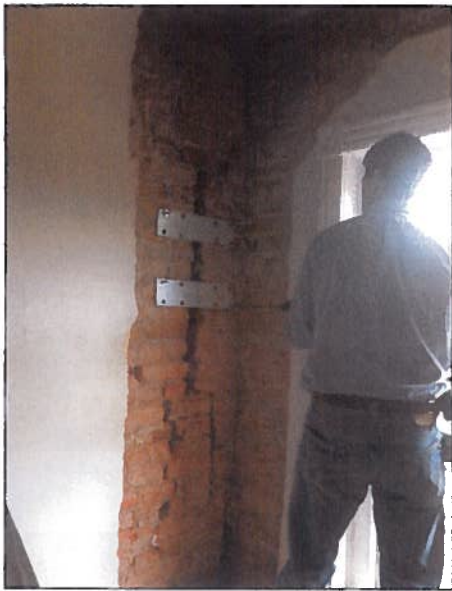
Photo 3: Cracks filled with spackle could not withstand last summer's earthquake. Temporary supports applied.
