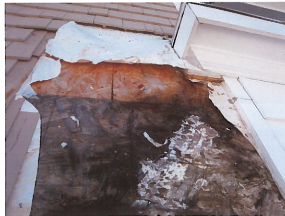
Water damaged wood sheathing under building wrap
