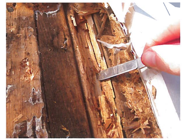
Decayed wood under the facade.
