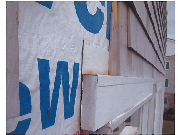
Window head flashing on top of house wrap and not under it.
