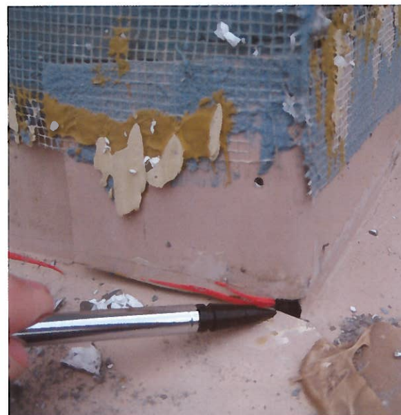
Unsealed window head flashing under EIFS
