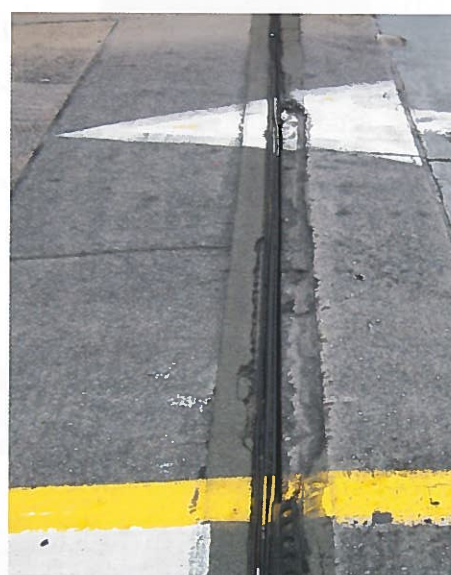
Snow plows often damage expansion joints
