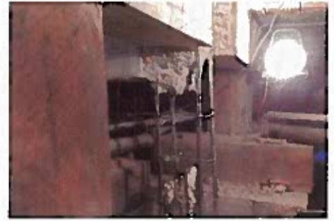
Figure 3: This photograph shows what is left of a concrete columns after all deficient was removed.
