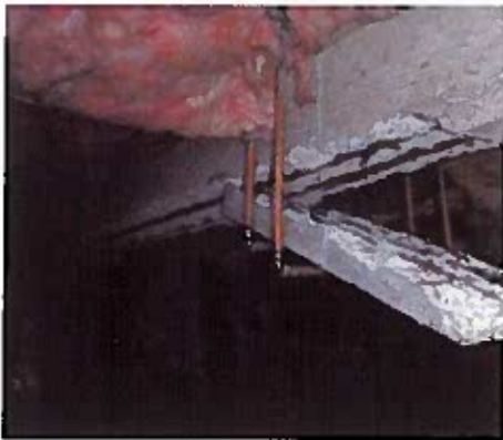
Figure 1: Typical damage to the concrete members found during the engineer's condition survey.
