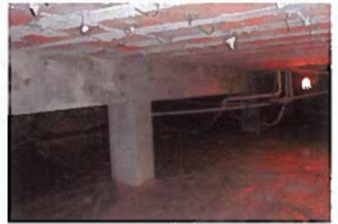
Figure 4: The crawlspace was cleaned and covered with plastic sheeting following the repairs to the concrete members.
