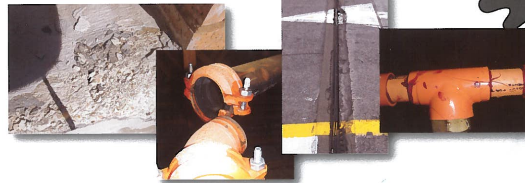
Photos of typical winter damage. From left to right: crumbling concrete, damaged steel sprinkler pipe, expansion joint damage, damaged lastic pipe
