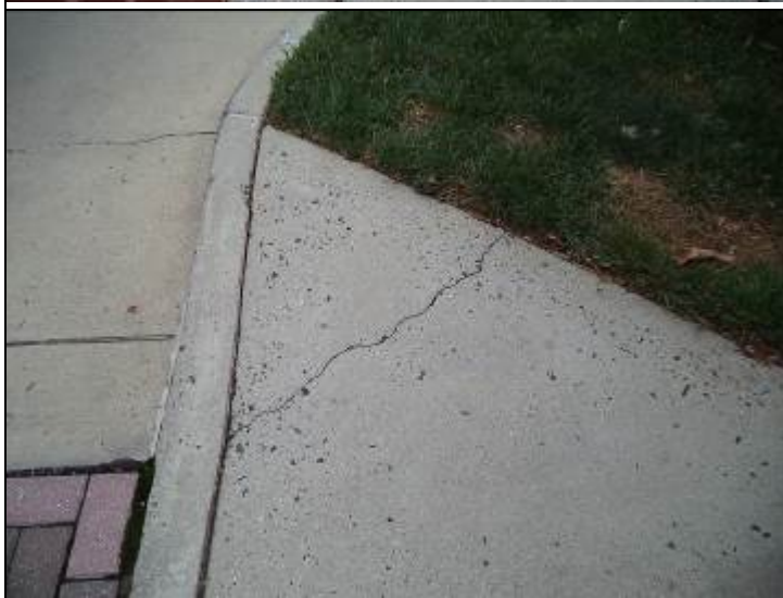
Photo #6: Minor walk cracks should be sealed.
