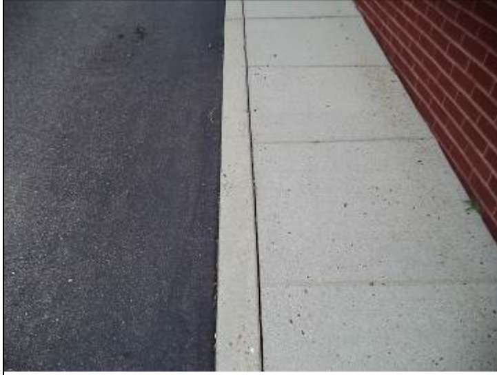
Photo #10: The joint between the walks and curbs should be sealed to prevent damage to the sub-base.
