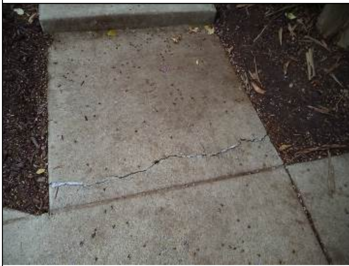
Photo #12: Minor walk cracks should be sealed.
