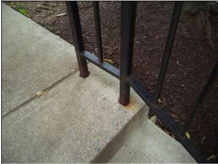
Photo #11: Consideration should be given to sealing the walk railing bases to keep ponding water from deteriorating the metal bases.
