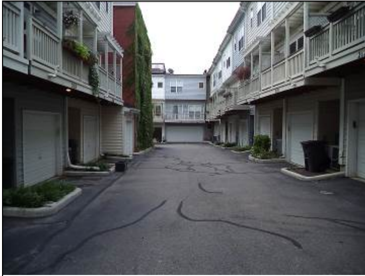
Photo #1: Asphalt surfaces are being maintained in good order crack fillings prevent extensive damages
