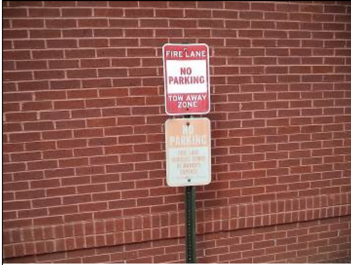
Photo #4: Signs are beginning to fade. Consideration should be given to replacing signs as needed.
