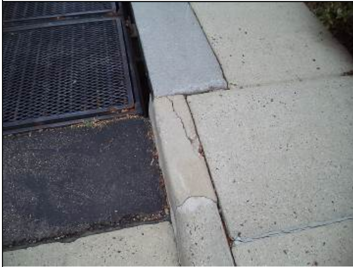
Photo #8: Minor walk cracks should be sealed.
