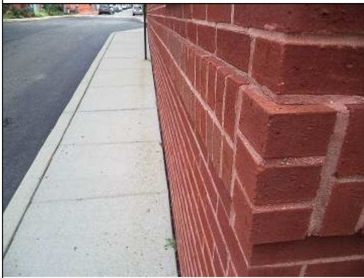
Photo #9: The joint between the walks and buildings should be sealed to prevent damage to the sub-base.
